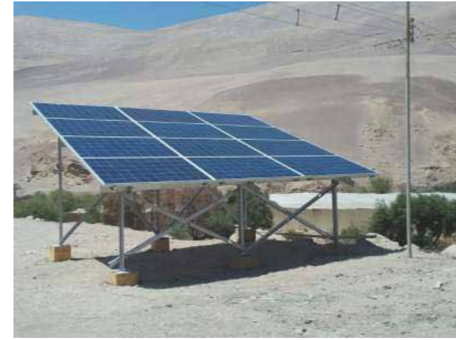
4 kW solar pumping system in Chile
