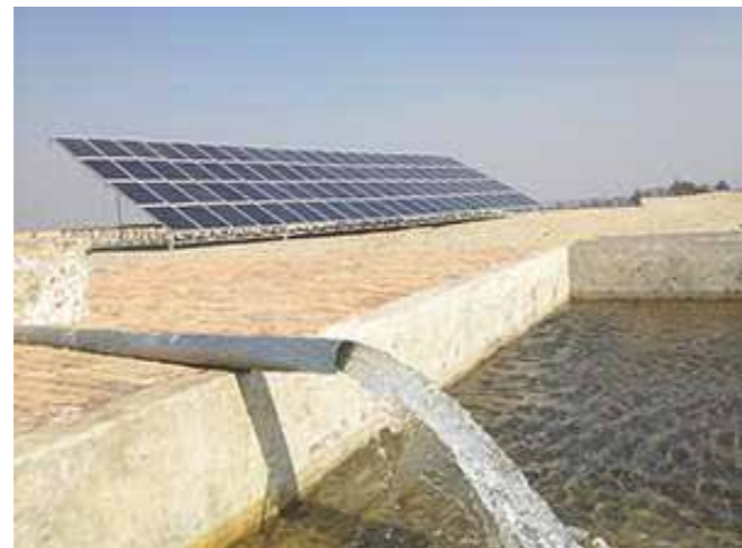
18.5kW solar pumping system in Pakistan
