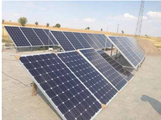
5.5kW solar pumping system in Turkey
