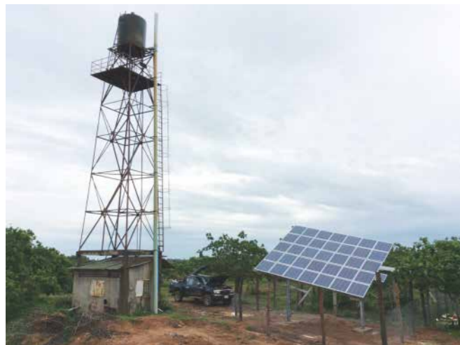
3.7kW solar pumping system in Cambodia
