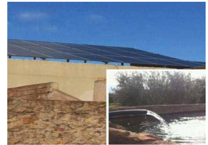
4kW solar pumping system in Morocco
