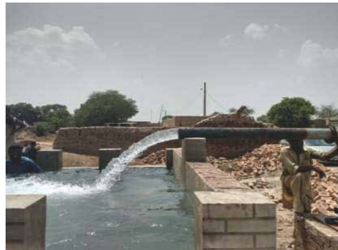
15kW solar pumping system in Pakistan
