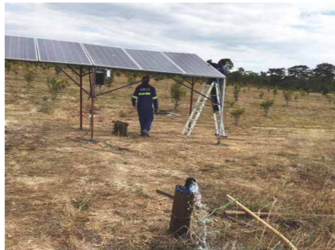
2.2kW solar pumping system in Zambia
