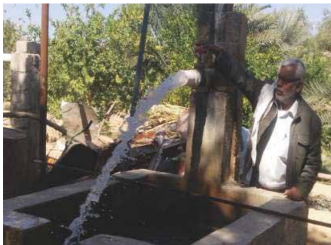
45kW solar pumping system in Yemen
