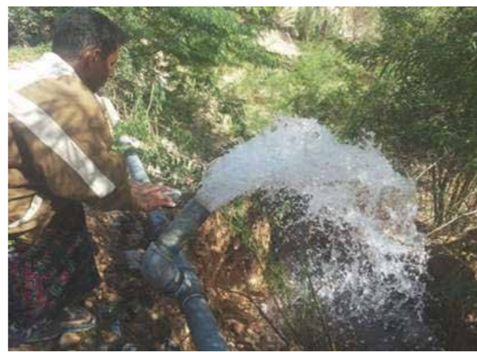
45kW solar pumping system in Yemen
