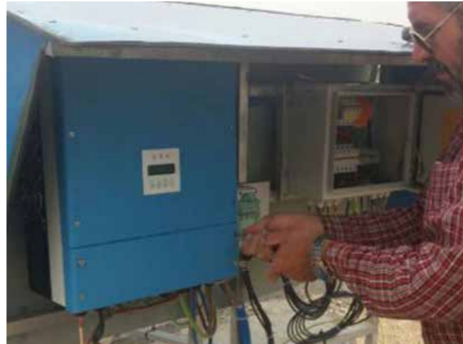
5.5kW solar pumping system in Jordan
