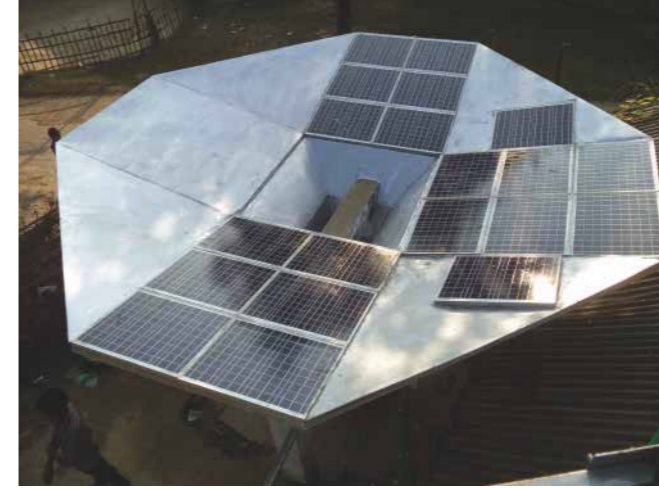
1.5kW solar pumping system in Bangladesh
