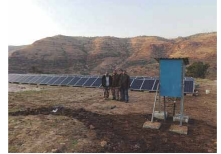
18.5 kW solar pumping system in Jordan
