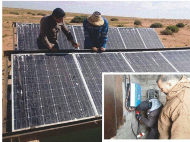
2.2kW solar pumping system in Algeria
