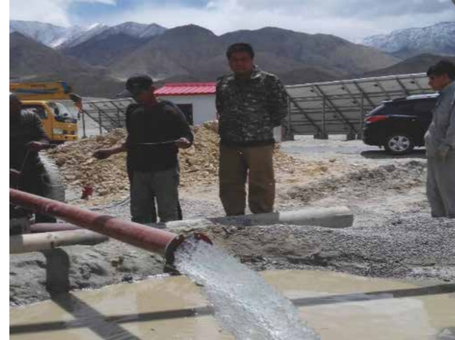
11kW solar pumping system in Xinjiang China
