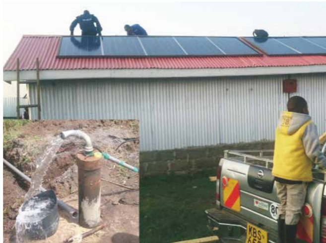
3kW solar pumping system in Kenya
