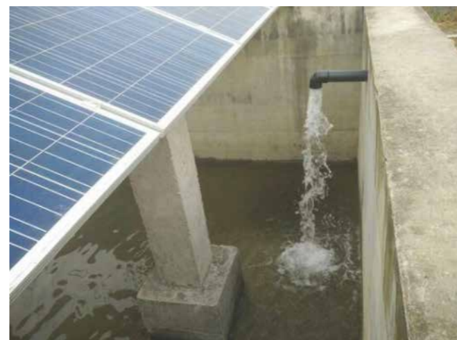
7.5kW solar pumping system in Jiangsu China
